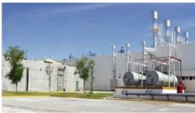
Data Center Triara Apodaca
